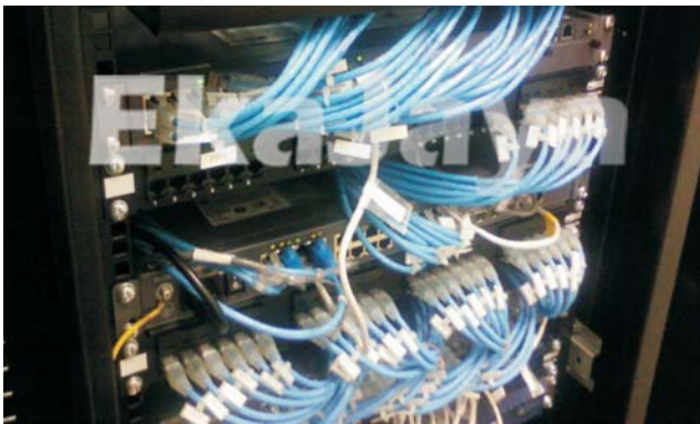
Data Cabinet Cabling w/ Switch - Patch Panel
