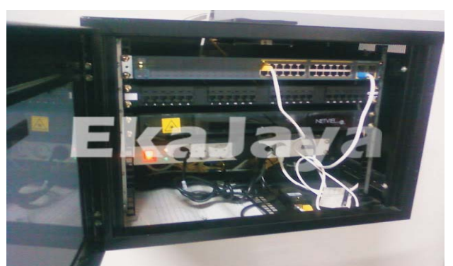
Distribution Rack : FO & Cat6 panel, data switch
