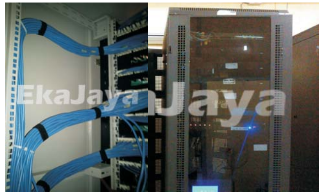
High density cabling @ cabinet data center
